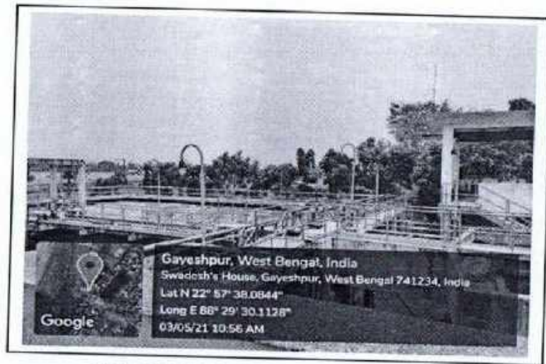
GAYESHPUR SBR-Aeration and filling
