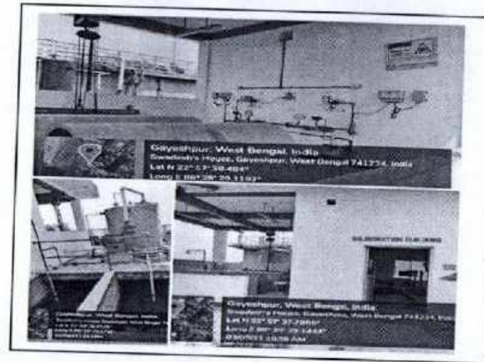
GAYESHPUR Chlorination system
